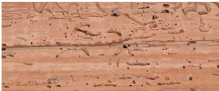
Figure 13 – Powder-post beetle damage
