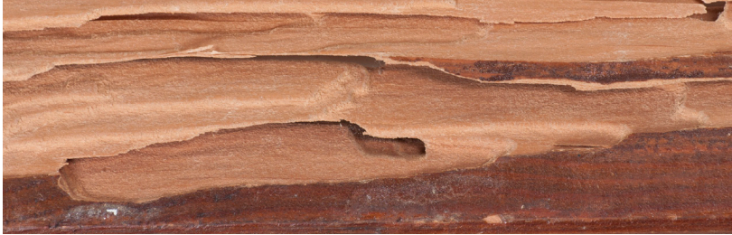
Figure 11 – Carpenter ant damage
