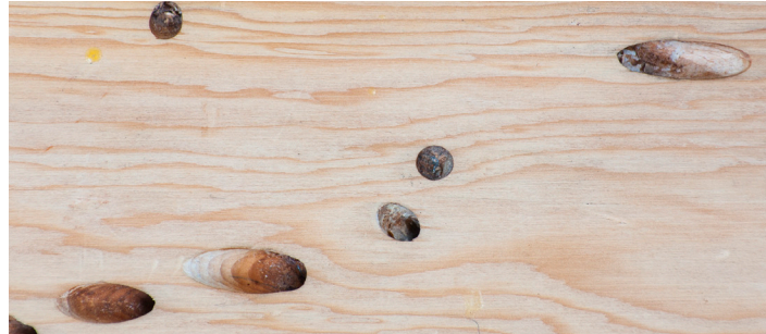
Figure 14–Teredo worm tunnel damage
