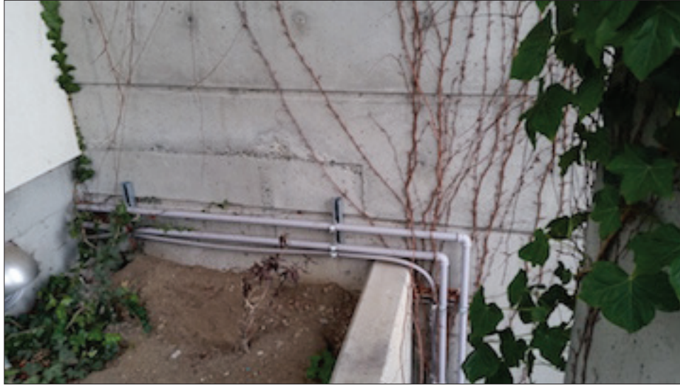
Figure 2 — The result of improperly aligned seams
