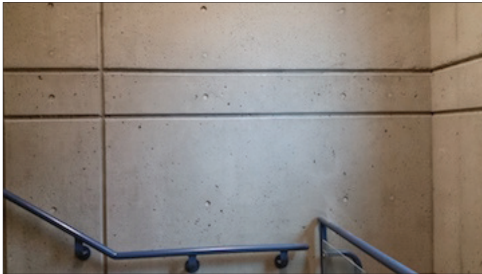
Figure 5 — Plugged tie holes
