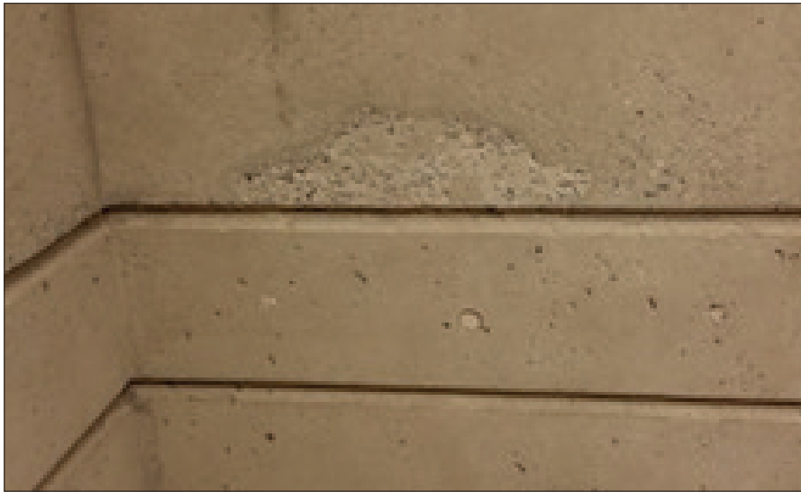
Figure 17 — Poorly patched architectural concrete
