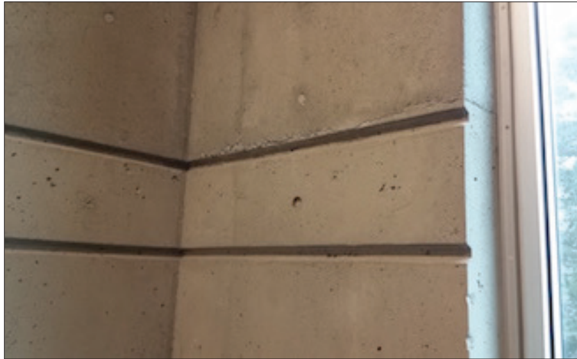
Figure 10 — Out-of-level rustication strip
