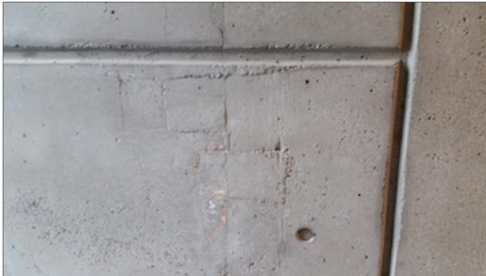
Figure 3 — The result of improper patching of forms
