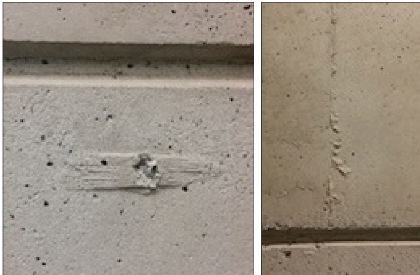
Figure 19 — Telegraphed form damage
