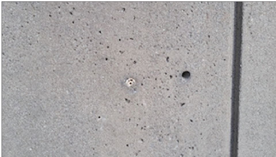
Figure 6 — Improper tie spacing with one cone left in place
