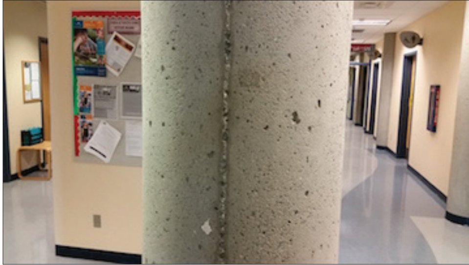
Figure 22 — Seam enlarged due to poor scraping and cleaning
